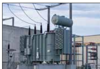
real image of a transformer
